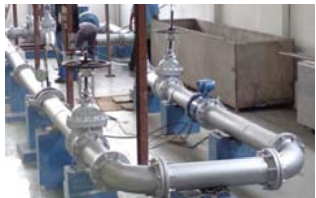
Radial metering system with calibrated pressure gauge, magnetic flow meter and DP gauges
